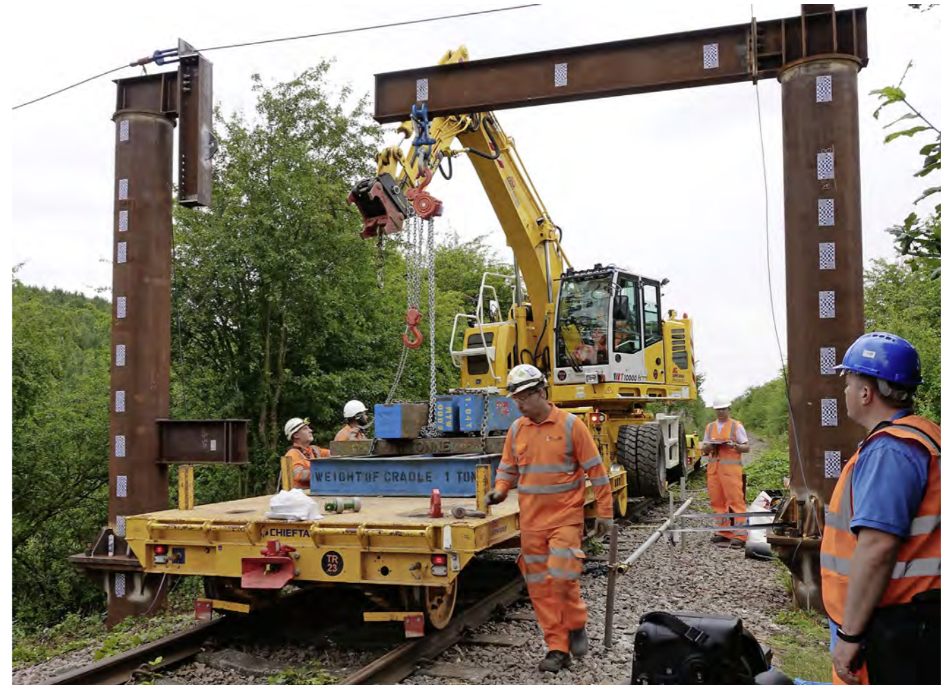
OLE foundation testing takes place at Network Rail's Rail Innovation & Development Centre (RIDC) at Tuxford, Nottinghamshire. It forms part of UKRRIN's Centre of Excellence in Testing alongside NR's RIDC at Melton Mowbray, Leicestershire, Transport for London's test facilities at Acton and Stratford and the Quinton Rail Technology Centre at Long Marston, Warwickshire. UNIVERSITY OF SOUTHAMPTON.
