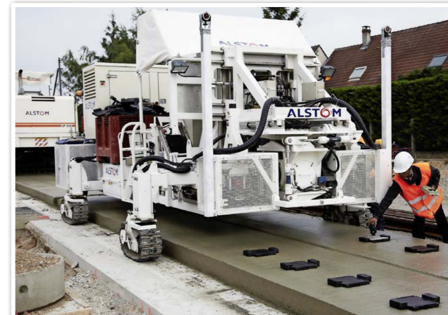
Nottingham Express Transit is where Alstom's Appitrack automated track laying system made its UK debut, in 2014, accelerating the laying of track by three to four times the normal rate. ALSTOM.
