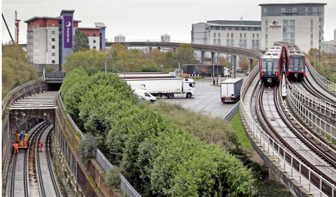
The scene at Prince Regent on August 10, where DLR trains arrive and depart beneath a British Airways plane taking off from London City Airport. To the left, work continues on the approach to Connaught Tunnel beneath the Royal Docks on Crossrail's south-eastern branch to Abbey Wood, due to open in December 2018. ANTONY GUPPY.
