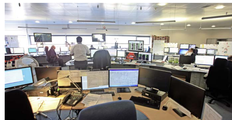
The DLR's Automatic Train Control (ATC) system is controlled from a central control room at Beckton, using moving block signalling. ANTONY GUPPY.
