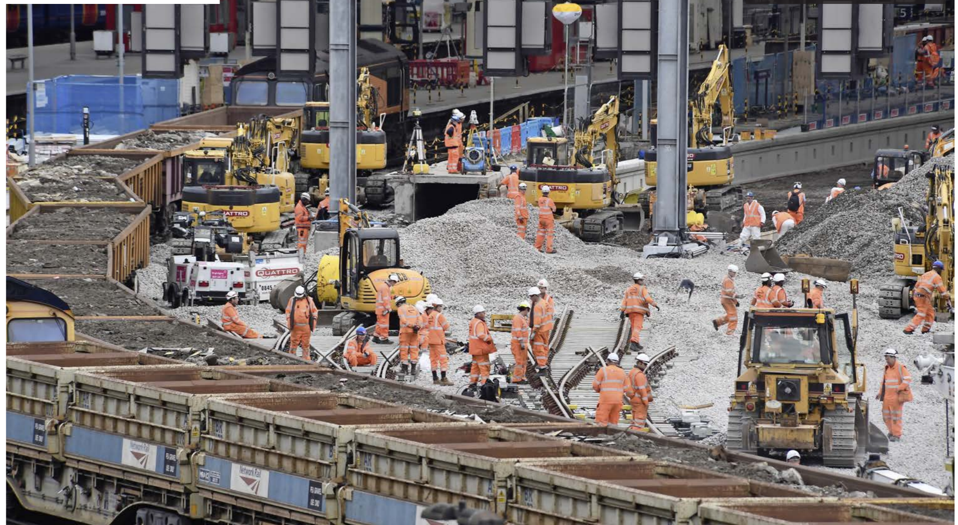
Four platforms were extended and more than a kilometre of new track laid during a 23-day partial blockade of Waterloo in August, demonstrating the power of alliancing. PAUL BIGLAND.
