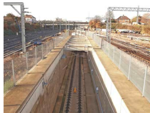
▲ Acton diveunder (above) has been built to reduce pathing conflicts between high-frequency Crossrail services and heavy freights in and out of Acton Yard. CROSSRAIL.
