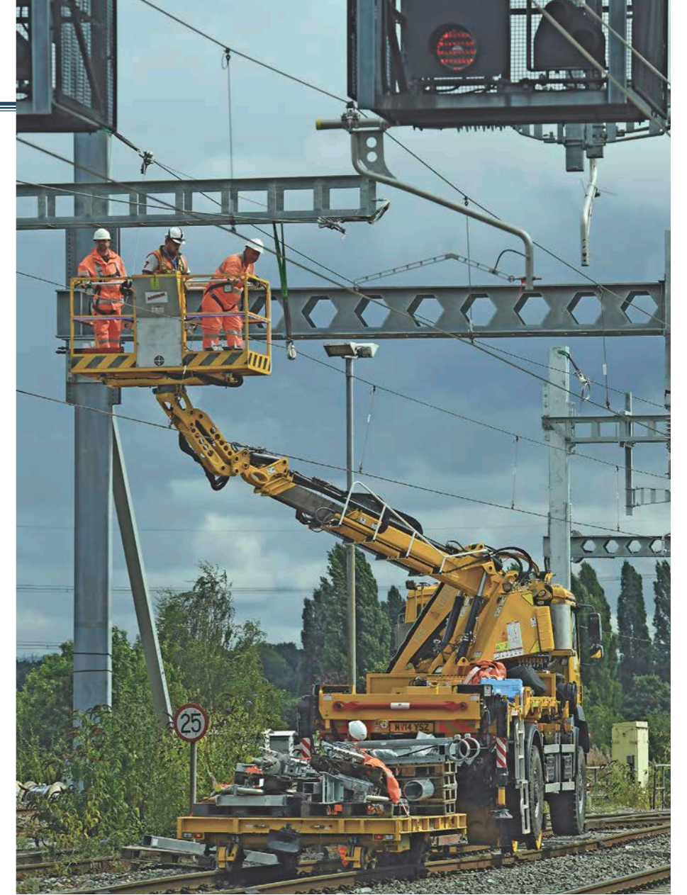
▲ Far from being an Achilles' heel, electrification and modernisation of the Great Western Main Line to Cardiff in the last 18 months has demonstrated the UK's capability to deliver. Engineers install overhead line equipment near Didcot. PAUL BIGLAND.
