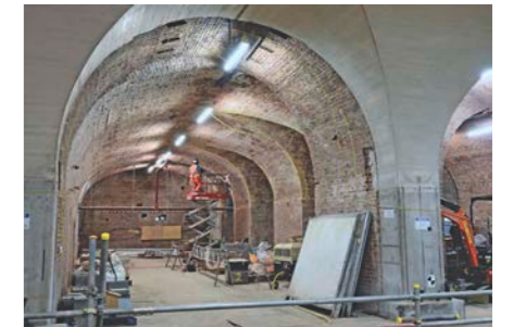
▲ The Grade II-listed St Thomas Street façade was retained and restored using specialist contractors with very pleasing results. Quadripartite arches were also retained and then replicated, demonstrating that heritage features can be altered sympathetically to deliver capacity enhancements. PAUL BIGLAND
