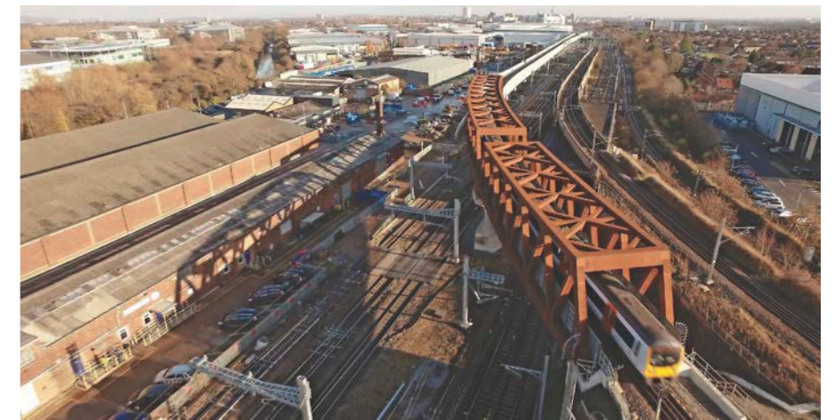
▲ Acton diveunder (left) and Stockley flyover (above) were both fully commissioned in December 2016 during NR's largest ever package of Christmas works. CROSSRAIL.
