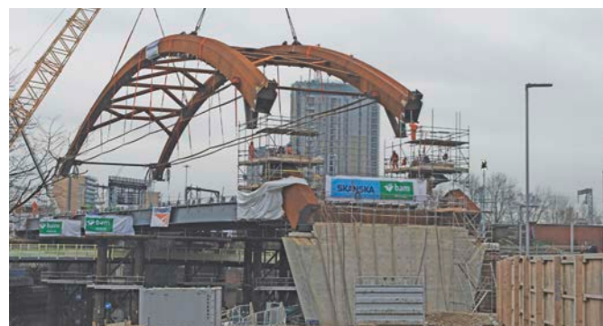
▲ Weighing 600 tonnes, the Ordsall Chord's signature network arch was fixed into position on February 21 having been constructed on site. PAUL STEPHEN.
