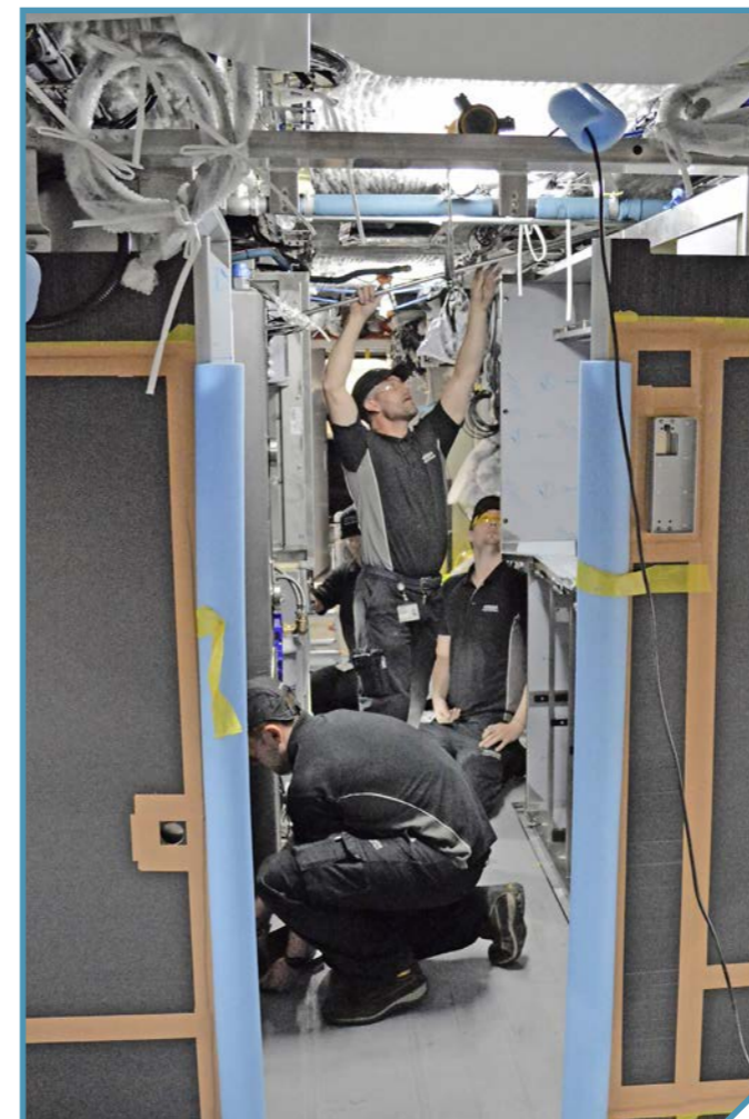
Above: Staff work on the fitting of a Class 800/3 kitchen at Newton Aycliffe. RICHARD CLINNICK.
