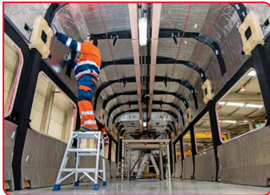
Inside a Talgo coach body during construction at Rivabellosa. The site in northern Spain is similar to how the company's Longannet factory will operate. TALGO.
