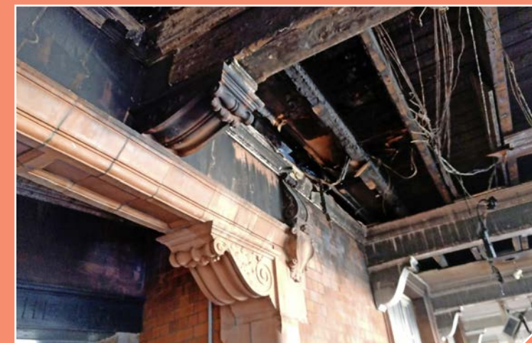
Repairs cost approximately £2 million, including the replacement of these charred wooden roof beams inside the main station footbridge. RAIL HERITAGE TRUST.
